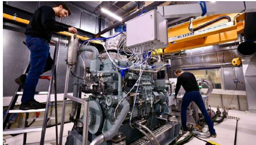
Maritime test cell 1.4 MW
